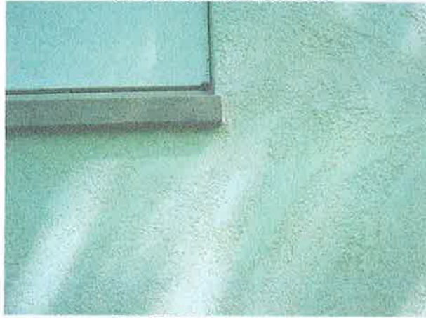
CRACKING AT REAR WALL
