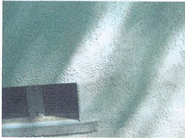
CRACK AT REAR WALL
