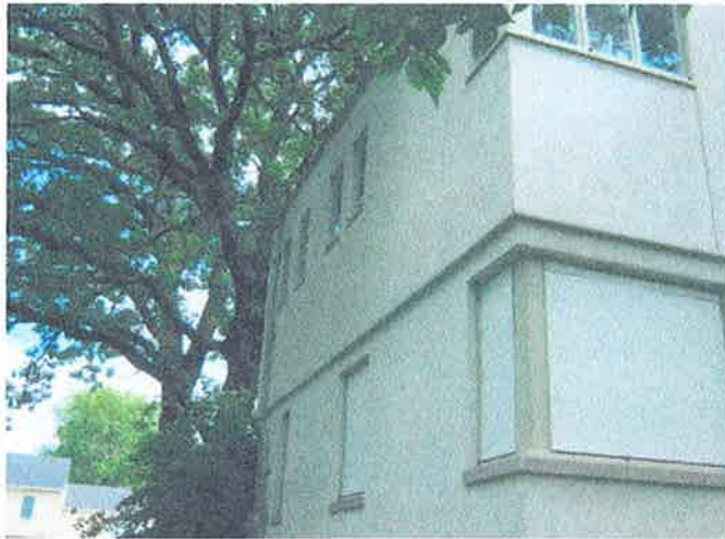
CRACKING AT CORNER
