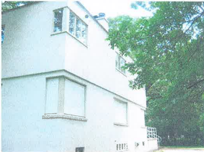
CRACKING AT CORNER
