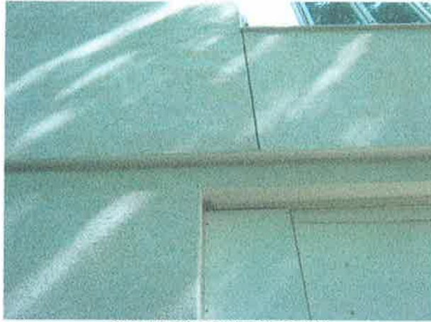
CRACKING AT THE CORNER
